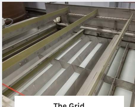
The Grid SLUDGE DEHYDRATOR
